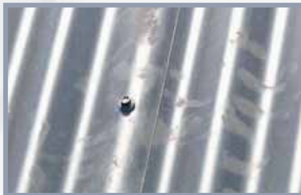
Fig 3. Finger marking damage to prepainted steel.
