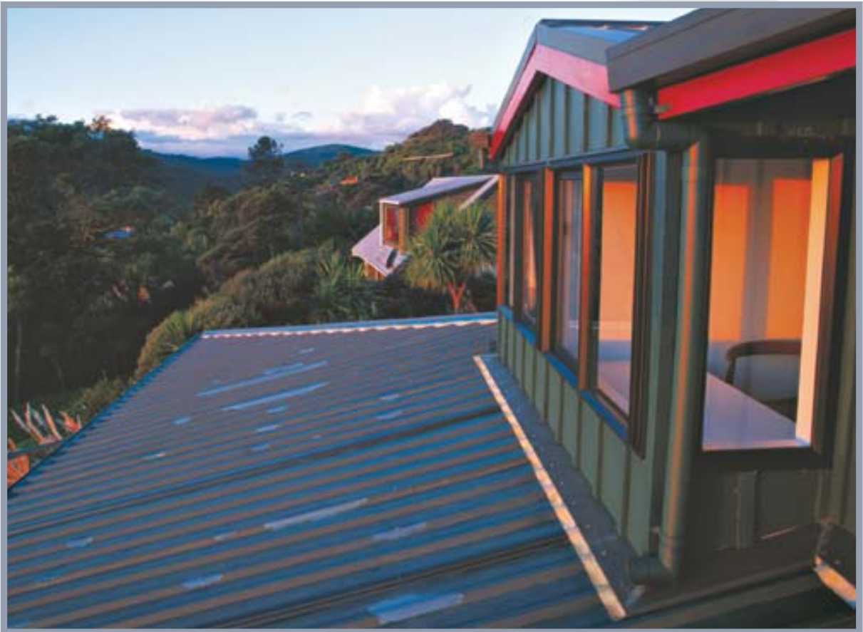
An extreme example of the overuse of touch-up paint. Damage caused by poor fixing is best dealt with by replacement of affected sheets.
