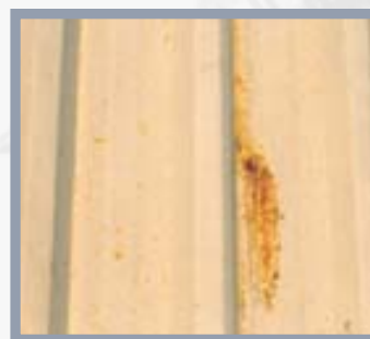
Typical swarf damage to COLORSTEEL® material.
